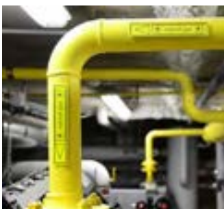
Pipes and valves identification
